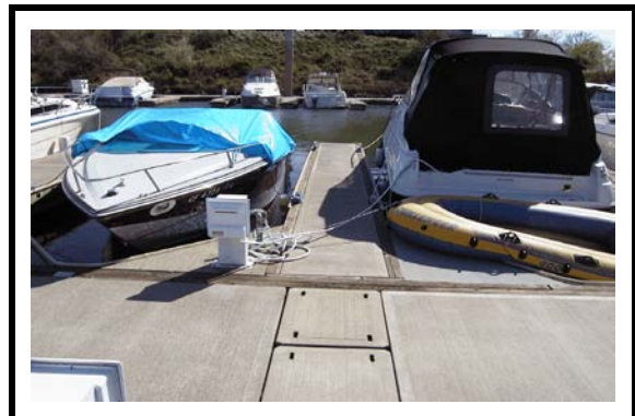
Non-Permanent Utility Lines Across Fingerfloat
