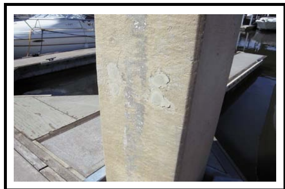
Rough Face on Square Concrete Pile
