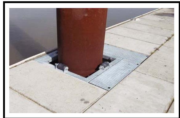
UHMW Rollers on Round Steel Guide Pile
